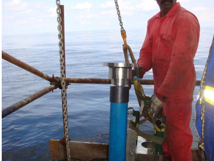
RTG flange that will be pushed back and flanged off the existing pipe
